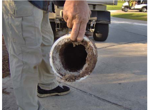
Cross sectional view of build up inside pipe
